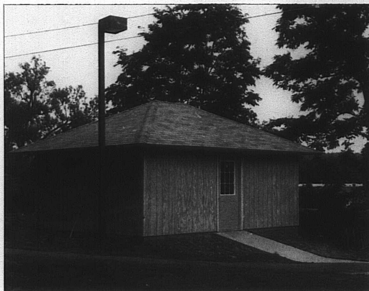
Right: the bike shed in the final stages of its construction. Photo Rocha 1991
